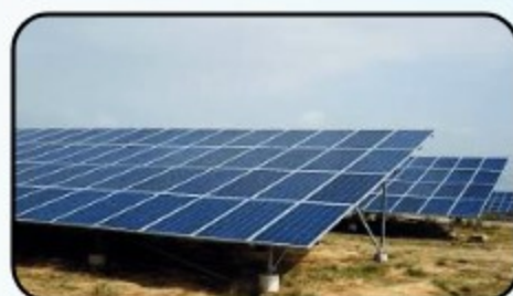
GROUND MOUNTED SOLAR (OPEX) PLANT
