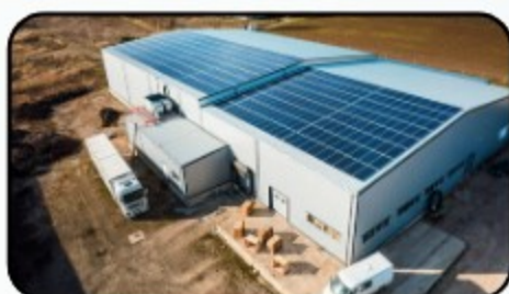
INDUSTRIAL SOLAR ROOFTOP
