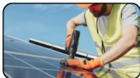
COMPREHESIVE SOLAR PLANT AMC
